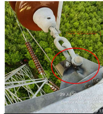
Loc 180 of 220 kV Misa Dimapur-1 dtd 29.07.2026
