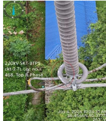
Loc 468 of 220 kV Salakati BTPS-2 dtd 03.06.2026
