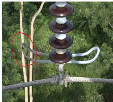
Loc 287 of 220 kV Misa Kopili-1 dtd 22.08.2026
