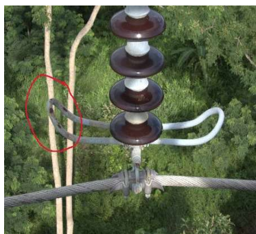
Loc 287 of 220 kV Misa Kopili-1 dtd 22.08.2026
