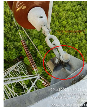
Loc 180 of 220 kV Misa Dimapur-1 dtd 29.07.2026
