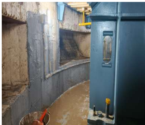
Inside Generator Barrel
