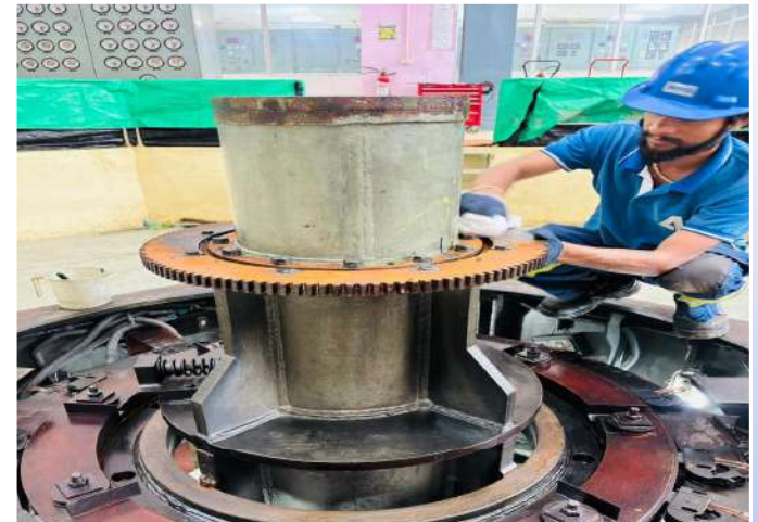
Cleaning of Slip Ring
