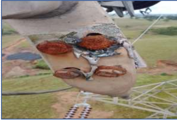
Before rectification (burned of jumper cone)
