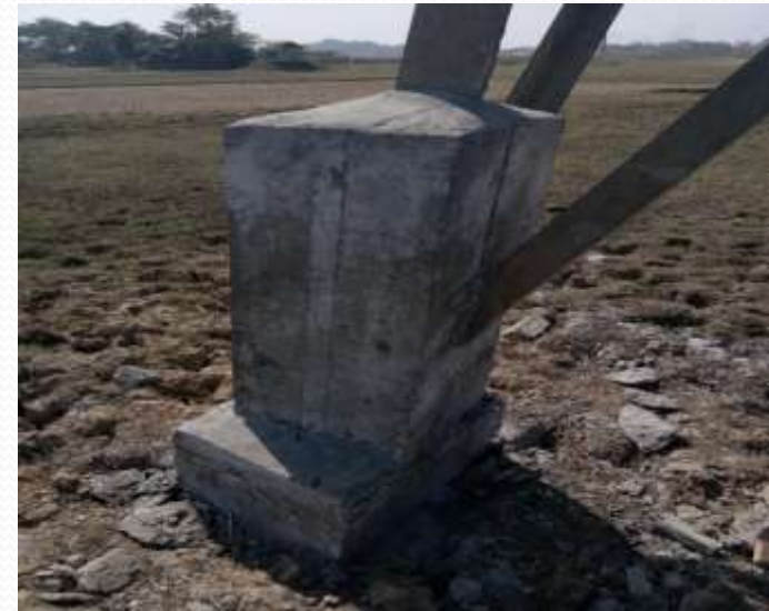
Stub encasement work for protection of tower legs and bracing members for water logged towers (During monsoon).
