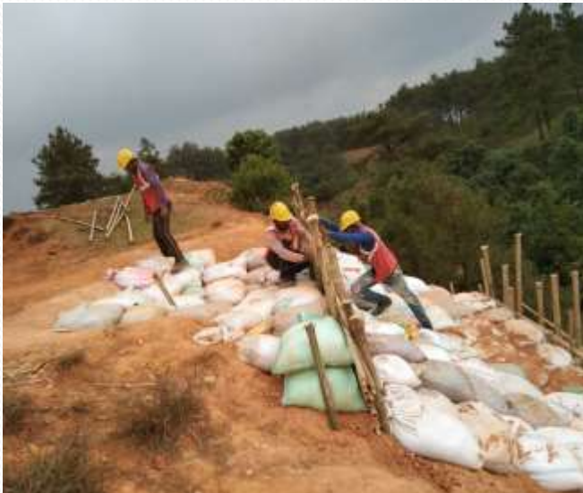
Temporary protection wall to avoid further soil erosion around the tower leg.
