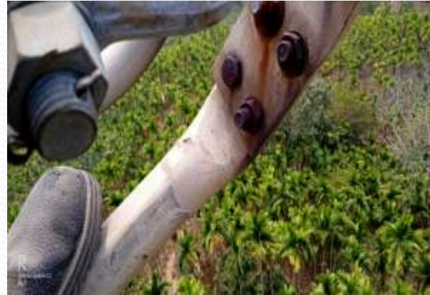
Before rectification (Rusted jumper N&B)
