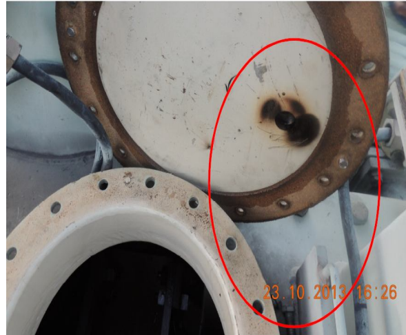
CARBON MARK ON TOP INSPECTION COVER (HV SIDE)
