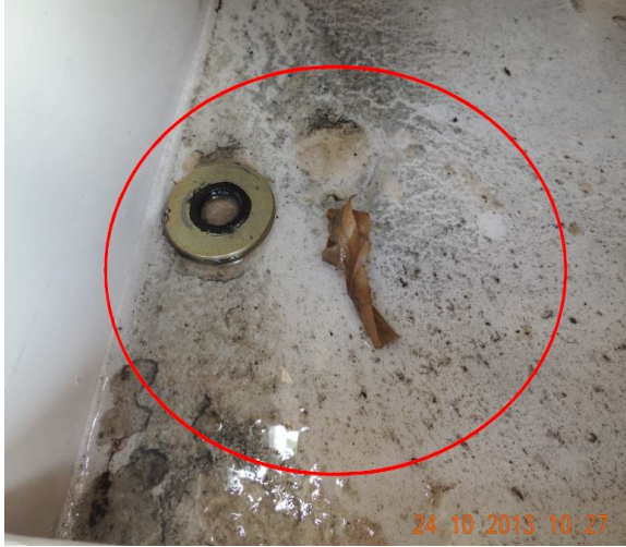
WASHER & PAPER FOUND NEAR BOTTOM INSPECTION COVER
