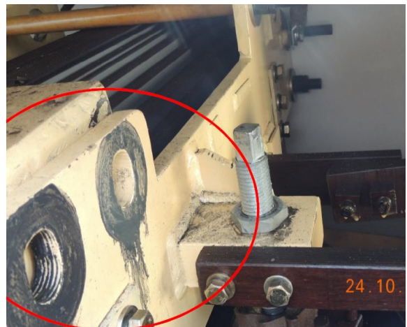
MISSING CLAMPING BOLTS (HV SIDE)
